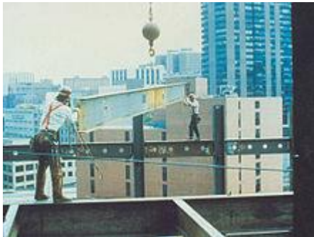
At-risk workers without appropriate safety equipment
