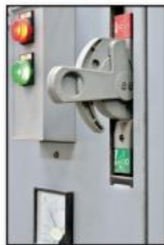
Main disconnect switch
