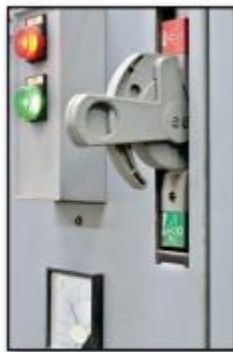
Main disconnect switch
