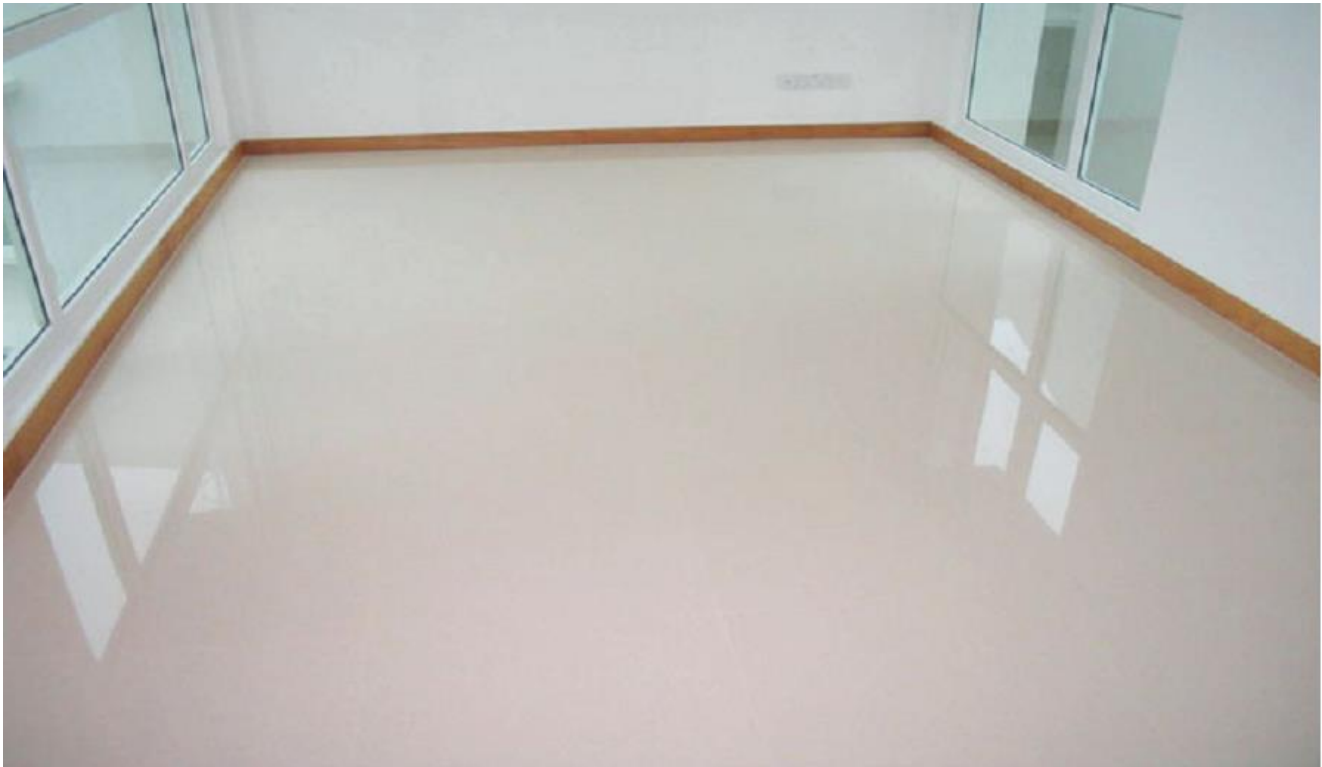
Fig. 9 – Better aesthetics and smoother joints on a marble floor using epoxy grout after polishing.
