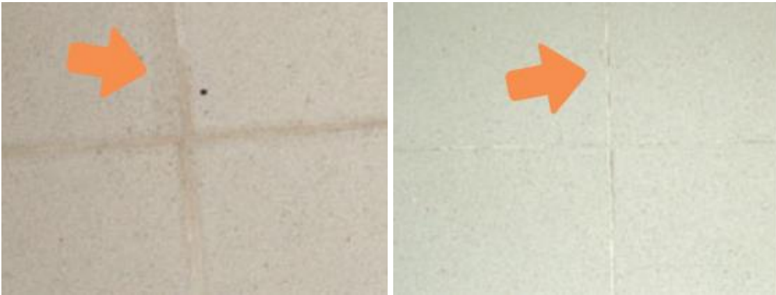
Fig. 6 – Discoloration of grout and edge Fig. 7 – Emerging grouts from marble joints.
