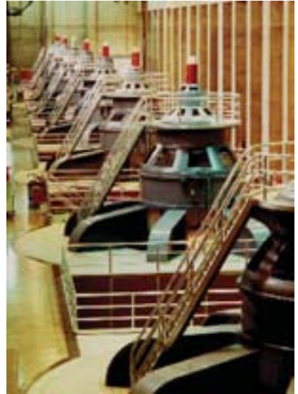
A series of hydel generators.
