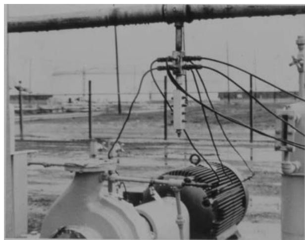
Figure 18-6. Open storage yard with oil mist tubing protecting pump and motor bearings.
